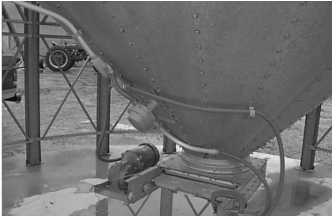
Wet Supply Rotary Switch Mounted on Wet Supply Tank
